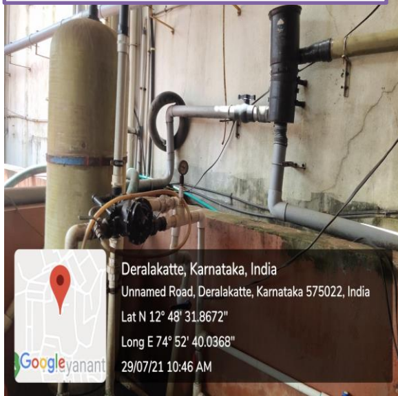
Borewell beside the Central Kitchen
